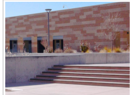
Exterior stair lacking handrails.
